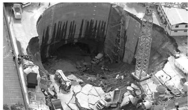
Figure 13. Air view of the collapsed tunnel and shaft.
